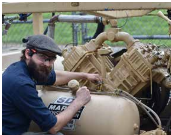
Kurt is working on a diesel-powered air compressor which supplies air to the divers. It can also be used to pressurize the hyperbaric chamber used to treat decompression sickness.
